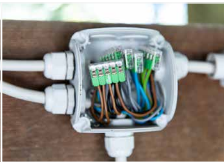
Wiring in the distribution box.
