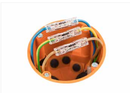
Wiring conductors in a flush-mounted junction box.
