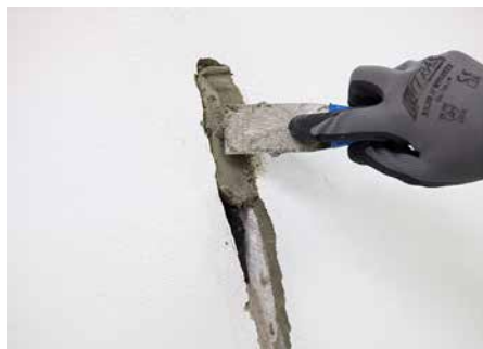
Close the damaged area discreetly.
